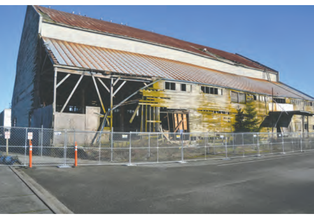
STILL DETERIORATING — The Moore-Clark warehouse is surrounded by temporary fencing in this 2022 file photo, but La Conner and Shelter Bay residents are concerned by the possible threats the building poses. — Photo by Ken Stern
