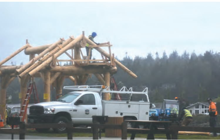
UP AND AT 'EM — La Conner Public Works Department employees install log rafters to the new pavilion they've been building at Conner Waterfront Park. — Photo by Madoc Hiller
