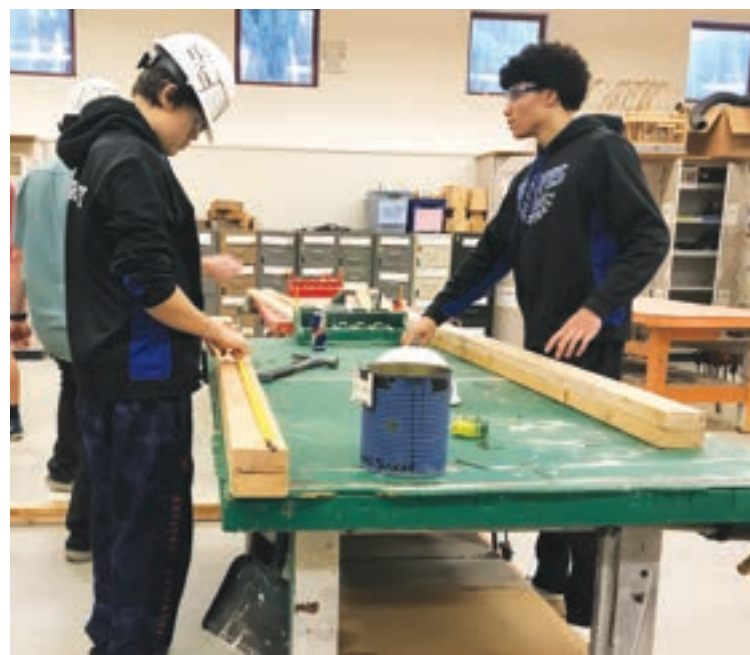
THESE STUDENTS ARE BUILDING A HOME – The 10 students in Daniel Castillo's La Conner High School construction class are building a tiny house to go in a tiny home village. – Photo by Madoc Hillier
