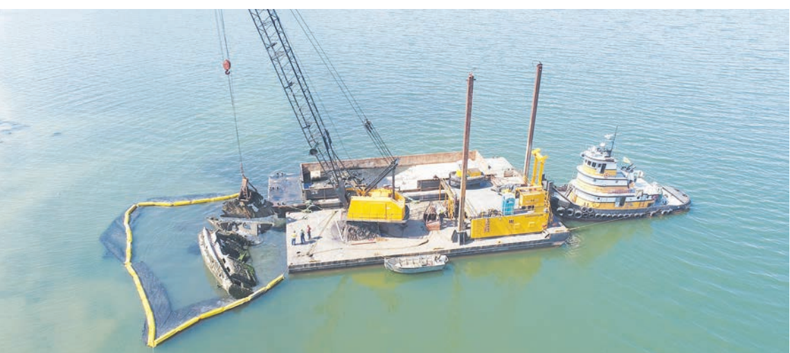
OUT OF HERE, FINALLY – A contractor working with the Swinomish Tribe and state agencies used a “demolition in place” method to remove portions of an abandoned sailboat in Similk Bay. A floating curtain was deployed around the sunken vessel to contain any turbid water.
