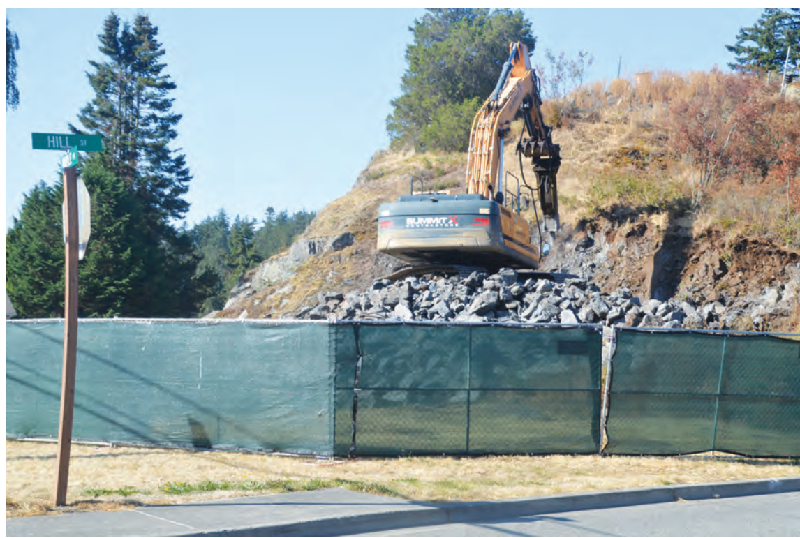
FUTURE SITE OF SNAPDRAGON FLATS – Excavating the base of Snapdragon Hill prepares the site for construction next spring of developer C.J. Ebert's Snapdragon Hill triplex apartment building. It will be followed by Snapdragon Park on the south side, another triplex. Story next week. – Photo by Ken Stern
