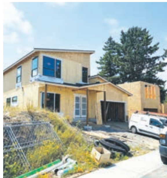
BUILDING UNABASHEDLY LUXURY HOMES – Construction of the first two homes in the La Conner Heights development began in early June. Developer BYK Construction has rebranded what has long been known as The Rock, or Snapdragon Hill. — Photo by Marissa Conklin
